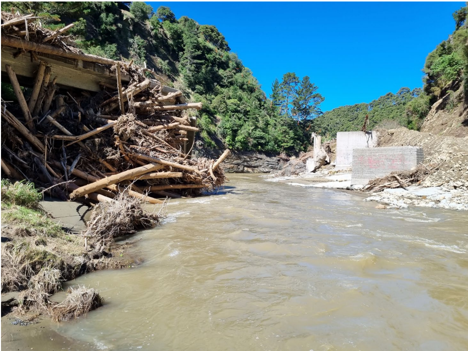
Figure 5: Broken State Highway 2 at Waikare
