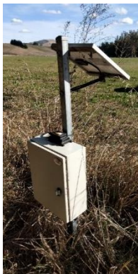
A solar-powered unit. The aerial is part of the small black box sitting on the bigger white box containing the logger.
