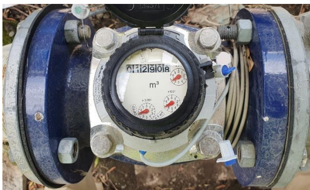
A mechanical water meter with a reed switch (grey cable at the bottom of meter), ready to be connected to a telemetry unit.
