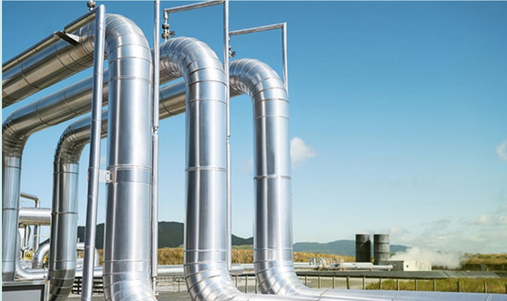
Image: Pipes at Ngā Tamariki geothermal station
