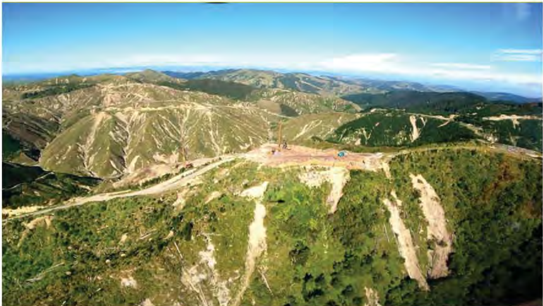
An example of a new-build landing that was in use by a cable yarding crew. Despite high construction standards and a relatively small footprint for such a large operation, there is still a slump right below the landing, a slip from the bench track on the left, and a slip most probably from the drainage as the road approaches the landing on the right.
