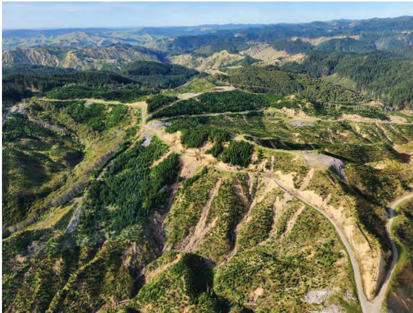
Pre-Labour weekend road and landing construction with many infrastructure triggered landslides evident, including from road and landing fill slopes
