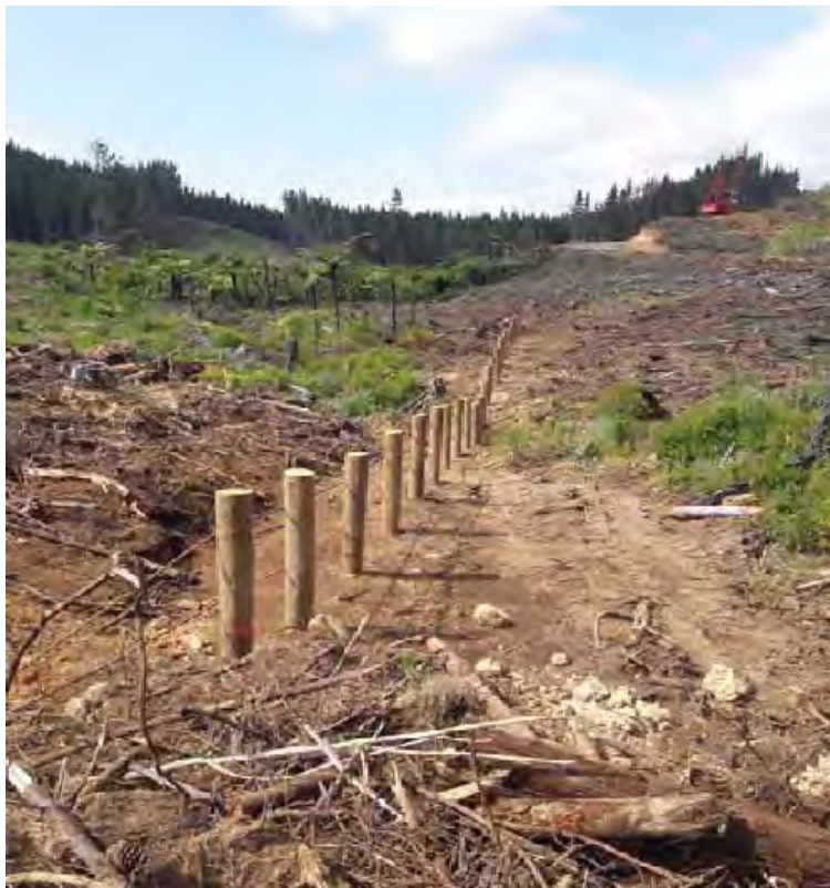
An example of a newly constructed trap using wooden posts. While also capable of trapping mobilised residues, its main design feature is to drive the residues from the main flow path onto the embankment where it can settle.
