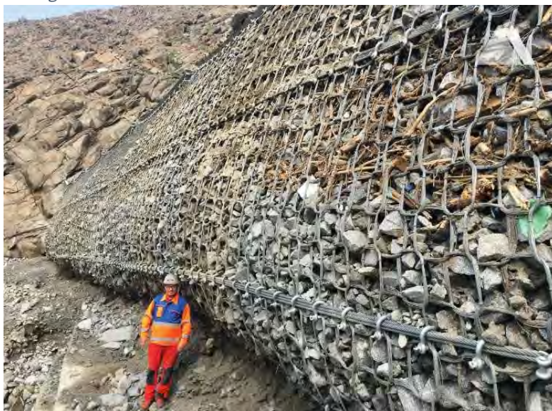
Figure 13 - Same barrier filled
