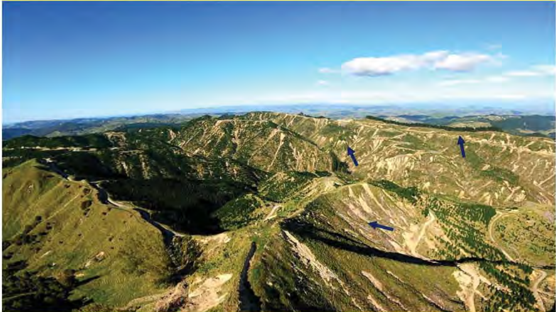
Infrastructure in the foreground has held up with minimal damage. However in the background there are many slumps / slips either onto the road or from the road (black arrows).
