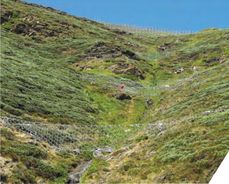
Figure 3 - Three debris barrier systems installed in Switzerland with low visual impact
