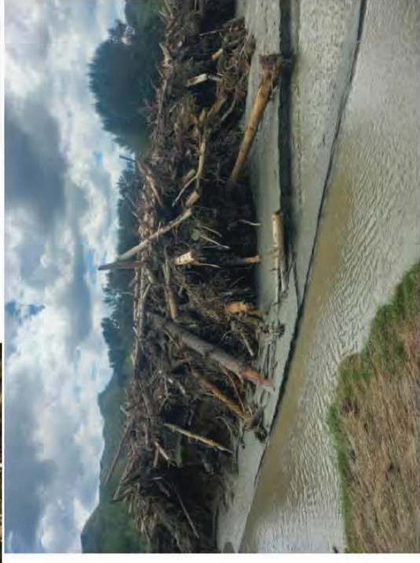
WR8 – Waimatā Valley 18km culvert. Mainly on true left bank of main river channel, downstream a few metres (WR9) piles are on both banks are c.3 metres in height.
