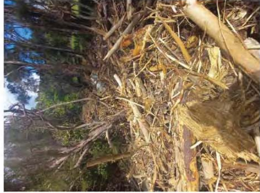
WR9 – Waimatā River, downstream from 18km mark culvert – 2+ metres deep in slash.
